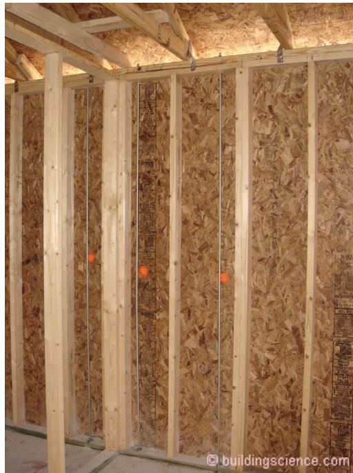
Photograph 1: Moisture Sensitive Materials - The newer materials are by and large more sensitive to water damage than the older traditional materials. Oriented Strand Board (OSB) is significantly more moisture sensitive than plywood.
