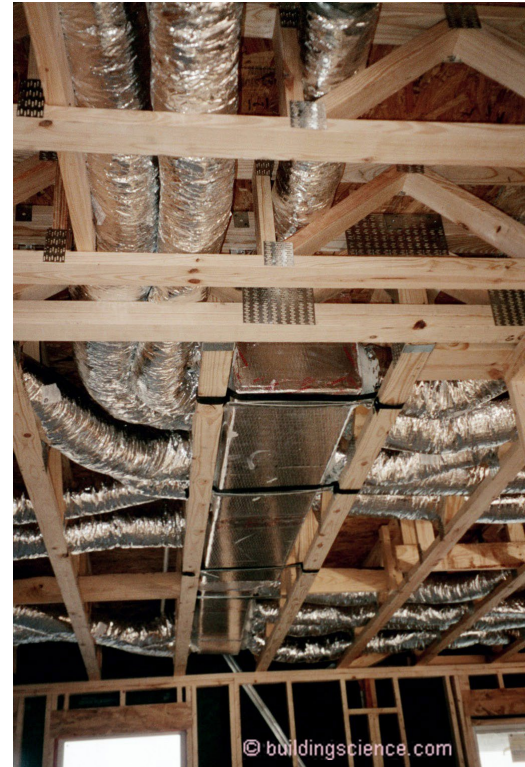
Photograph 3: Ductwork – Buildings now have ducted and fan-driven heating, cooling and ventilation systems and are significantly more airtight, so moving large quantities of air within them can lead to unacceptably high negative and positive air pressure differences.
