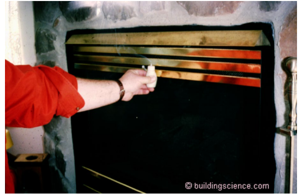
Photograph 5: Back-drafting Fireplace - Negative pressures due to air exhausting systems backdraft combustion systems such as fireplaces.
