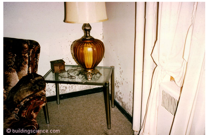
Photograph 6: Mold - When we caulked and sealed old buildings we reduced air change and increased interior mold.
