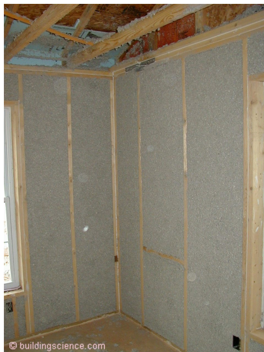
Photograph 2: Thermal Insulation - Significant increases in thermal insulation added to wall assemblies, roof assemblies, and foundation assemblies.
